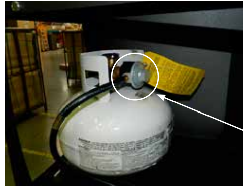
Gas connection @ tank
